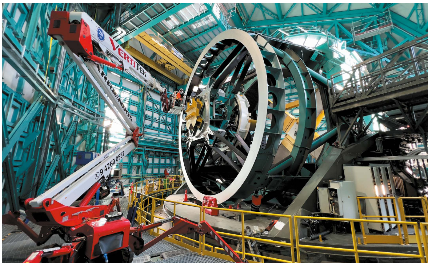
A technician installs fibre-optic cables at the Vera C. Rubin Observatory, which is due to take its first images in 2023.
